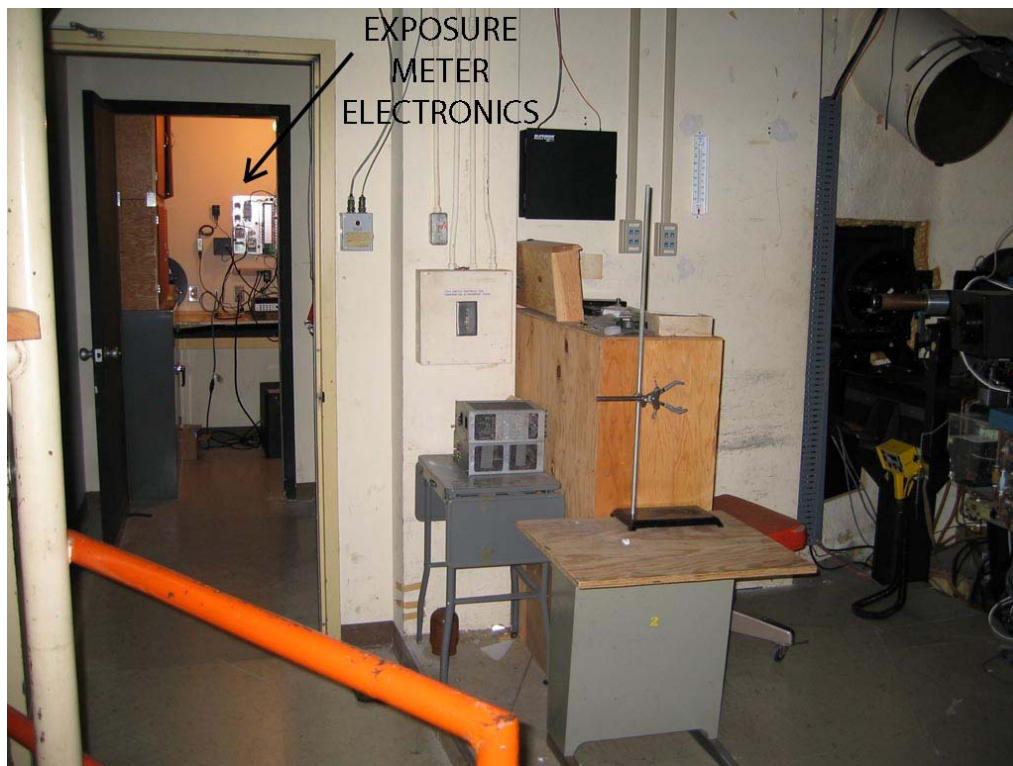
Figure 1: location of the exposure meter electronics relative in the 107" coude spectrograph area (taken before the slit room wall was installed).
